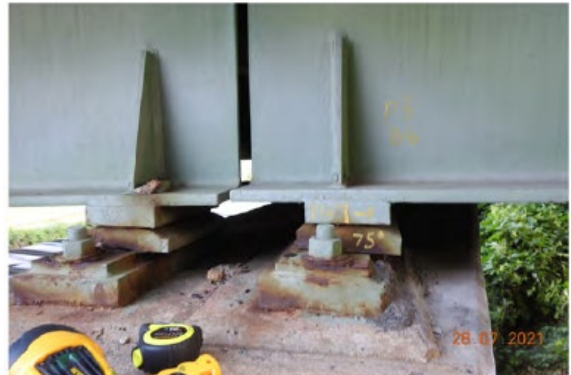
BRIDGE 13, PIER 3 UNIT 3, STRINGER 1-6 UNIT 4, STRINGER 5-6 BEARING MISALIGNED
