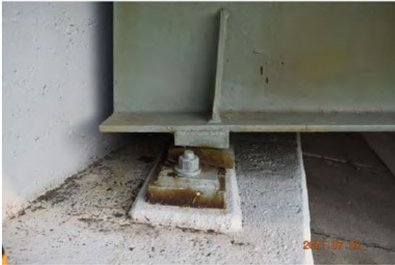
BRIDGE 13, WEST ABUTMENT UNIT 1, STRINGER 6 BEARING MISALIGNED
