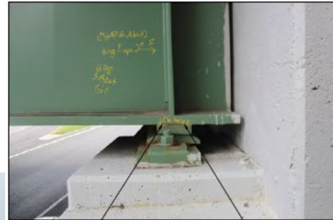
UNIT 1, GIRDER 1, SOUTH ABUTMENT BROKEN WELD REPAIR @ BEARING WEST FACE
