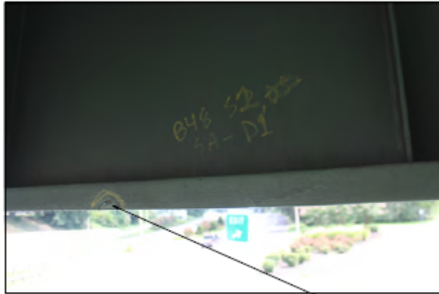
BRIDGE 48 UNIT 1, GIRDER 8 LAMINAR DEFECT
