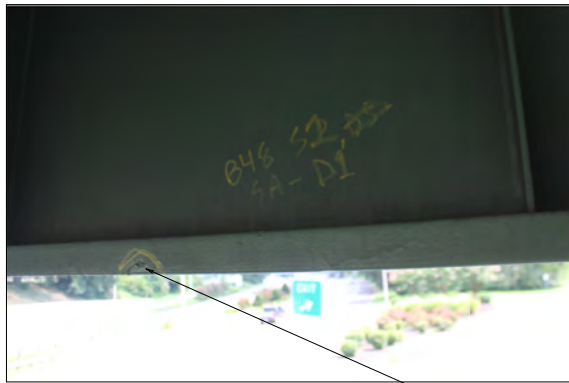
BRIDGE 48 UNIT 1, GIRDER 8 LAMINAR DEFECT
