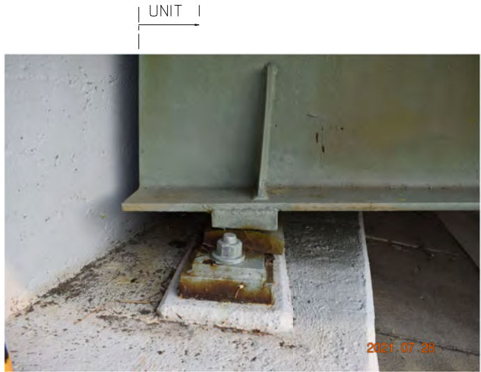
BRIDGE 13, WEST ABUTMENT UNIT 1, STRINGER 6 BEARING MISALIGNED
