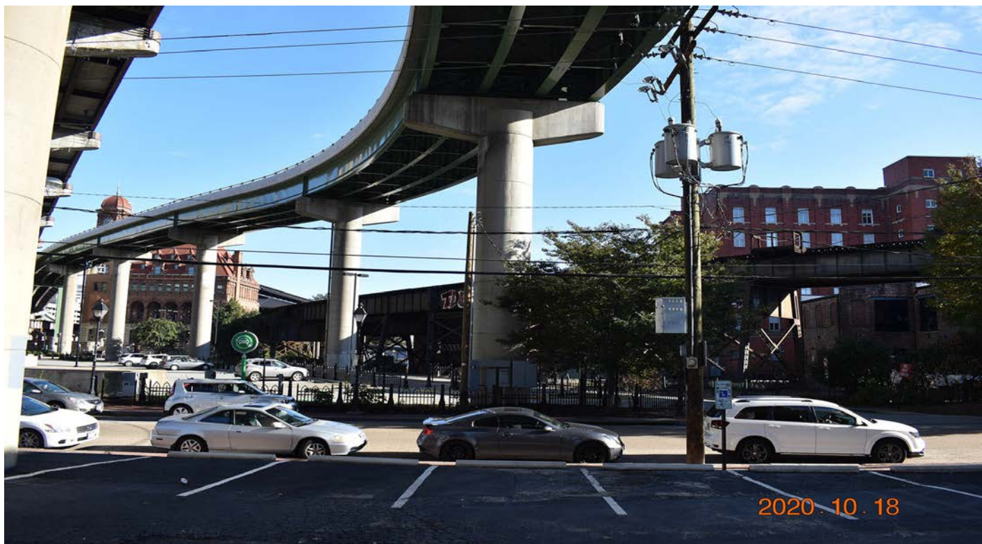
Ramp from EB DTE to NB I-95 over East Cary St, Dock St, East Main St and CSX railroad
