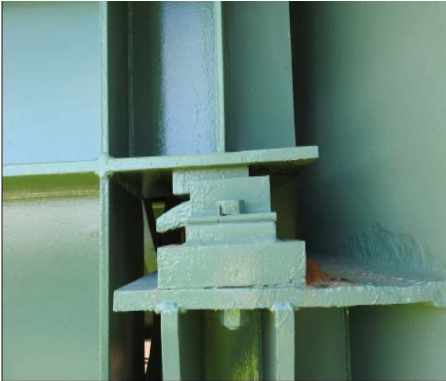
BRIDGE 66, PIER 16, SPAN 16 TYPICAL MISALIGNED BEARING
