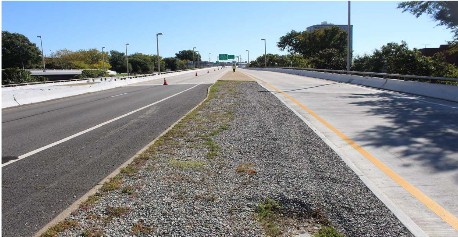
EB DTE over Virginia St, South 14 th St, South 12 th St and CSX
