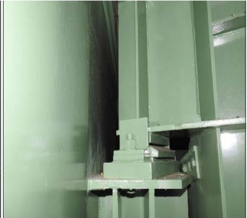
BRIDGE 66, PIER 19, SPAN 19 TYPICAL MISALIGNED BEARING
