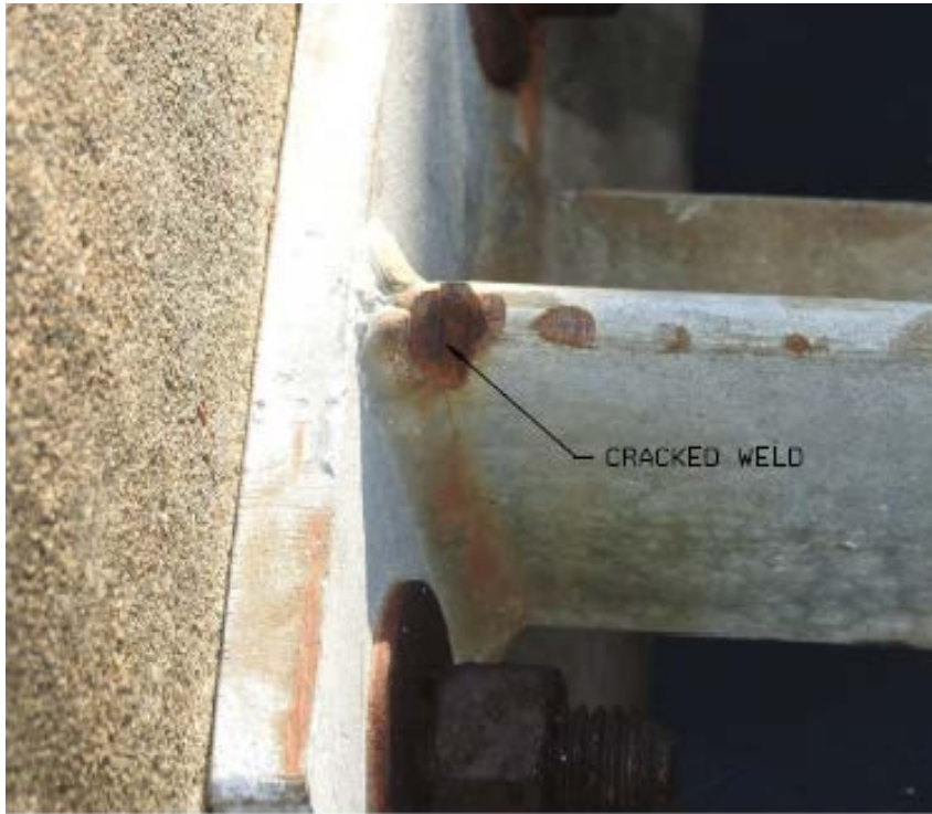
BRIDGE 13 SOUTH SIGN SUPPORT SOUTH FACE CLOSE-UP OF CRACKED WELD
