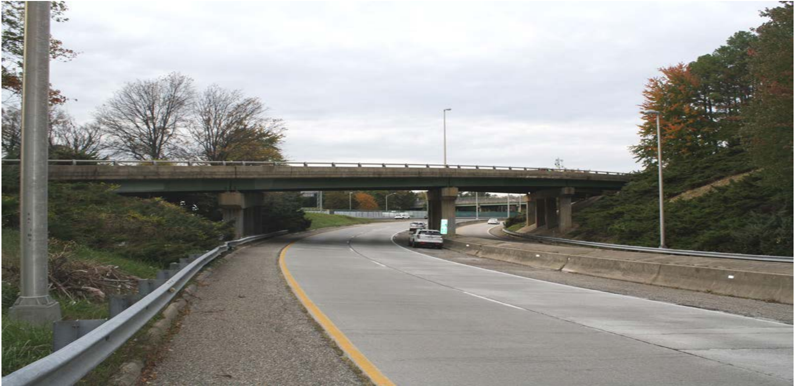
Ramp from NB Powhite Parkway/NB I-195 Connector over NB I-195 to Cary St and Ramp from NB I-195 to Floyd Avenue
