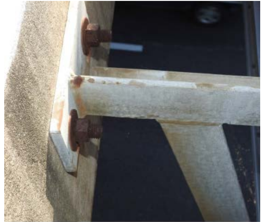
BRIDGE 13 SOUTH SIGN SUPPORT SOUTH FACE CRACKED WELD
