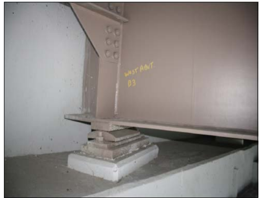
BRIDGE 62, WEST ABUTMENT TYPICAL GIRDERS 1-4 MISALIGNED
