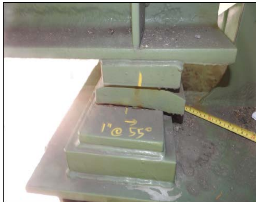
BRIDGE 67, PIER 13E, SPAN 14 SOUTH FACE, MISALIGNED BEARING
