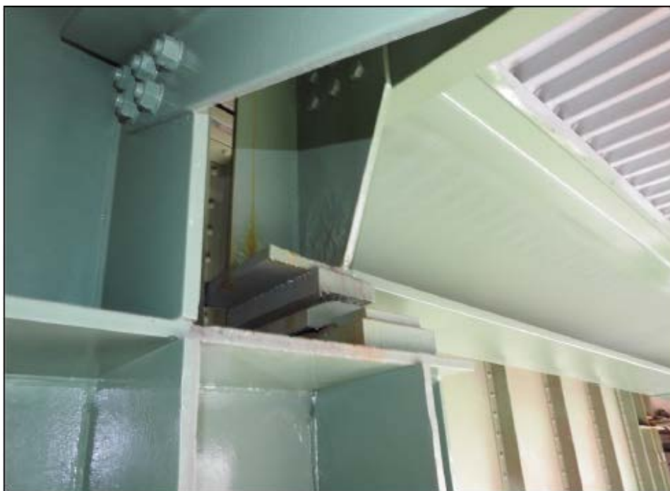
BRIDGE 67, PIER 13E, SPAN 14 SOUTH FACE, MISALIGNED BEARING
