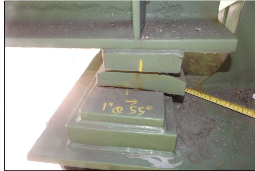
BRIDGE 67, PIER 13E, SPAN 14 SOUTH FACE, MISALIGNED BEARING
