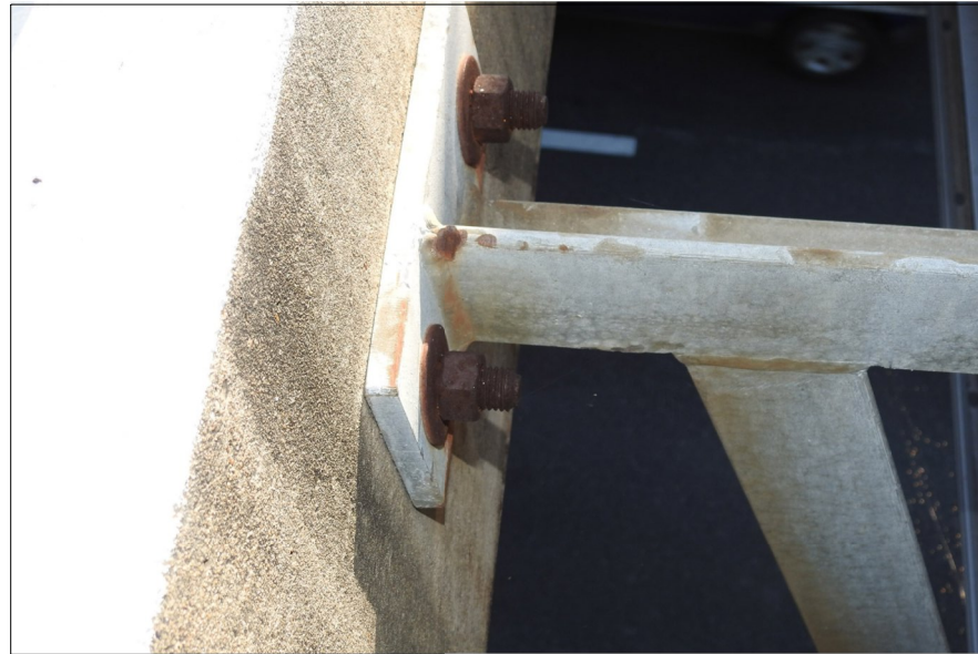
BRIDGE 13 SOUTH SIGN SUPPORT SOUTH FACE CRACKED WELD
