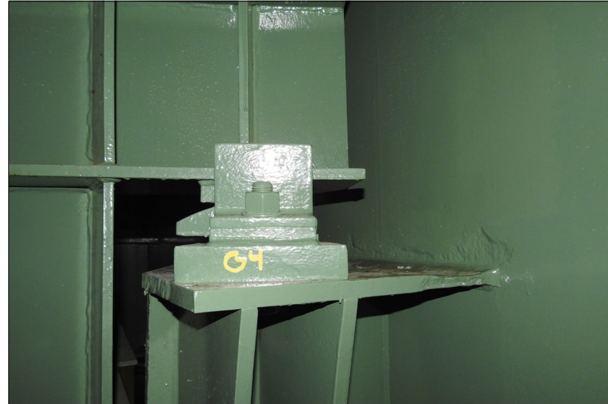
BRIDGE 66, PIER 19, SPAN 19 TYPICAL MISALIGNED BEARING
