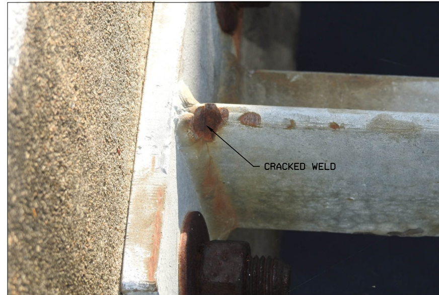
BRIDGE 13 SOUTH SIGN SUPPORT SOUTH FACE CLOSE-UP OF CRACKED WELD
