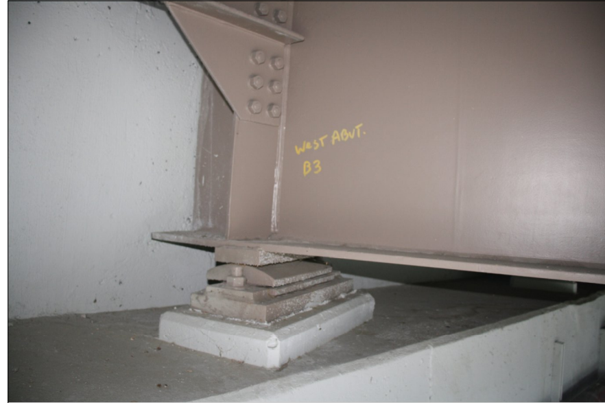
BRIDGE 62, WEST ABUTMENT TYPICAL GIRDERS 1-4 MISALIGNED
