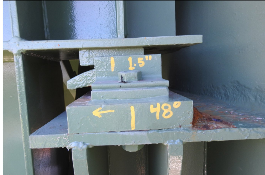
BRIDGE 66, PIER 16, SPAN 16 TYPICAL MISALIGNED BEARING
