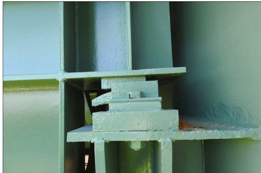
BRIDGE 66, PIER 16, SPAN 16 TYPICAL MISALIGNED BEARING
