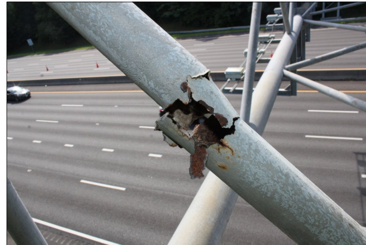
CLOSE-UP VIEW OF SECTION LOSS
