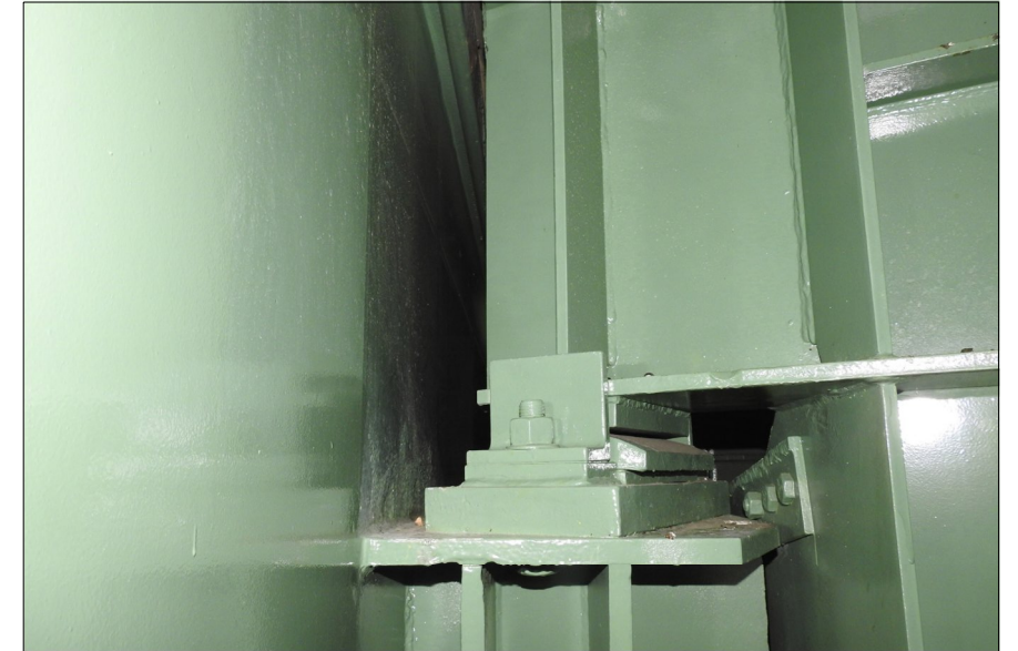
BRIDGE 66, PIER 19, SPAN 19 TYPICAL MISALIGNED BEARING
