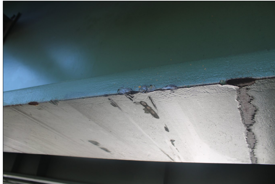
BRIDGE 47 SPAN 1, STRINGER 1 CLOSE-UP OF REPAIR 2
