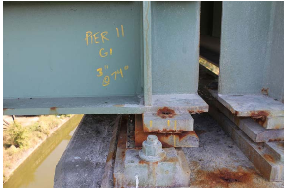
BRIDGE 65, PIER 11 STRINGER 1-12, BEARING MISALIGNED
