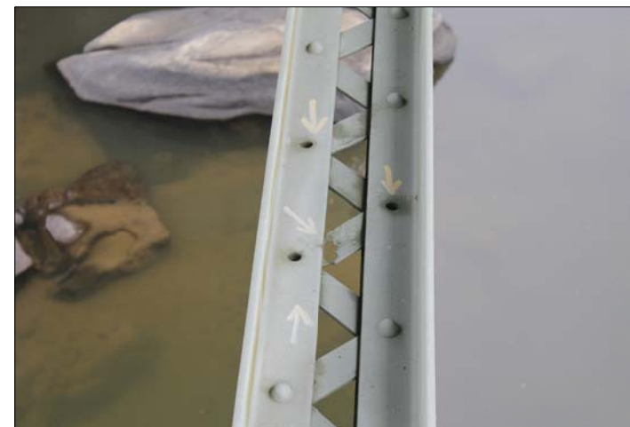
TYPICAL SECTION LOSS OF LACING BARS AND MISSING RIVETS ON TRUSS LOWER CHORD
