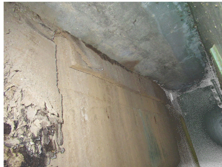
BRIDGE 8 - DECK SOFFIT AT SOUTH ABUTMENT PREVIOUS REPAIR CONCRETE CAST AGAINST BACKWALL
