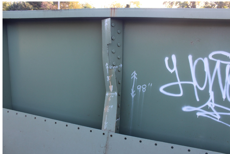
BRIDGE 9N - DAMAGED INTERIOR STIFFENER ON THROUGH GIRDER
