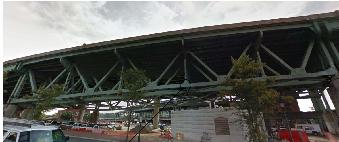
ELEVATION VIEW Location of Interior gusset plate repair (exterior gusset plate shown)
