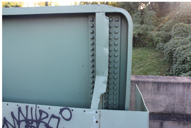
BRIDGE 9N DAMAGED BEARING STIFFENER MISSING RIVETS AT NORTHEAST BEARING
