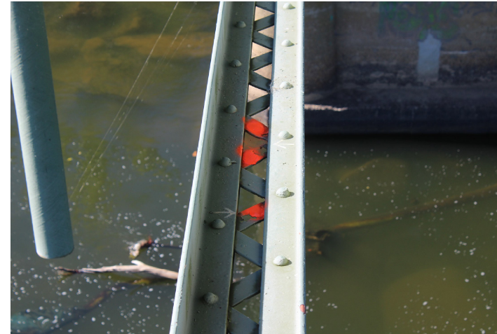
TYPICAL 100% SECTION LOSS OF LACING BARS
