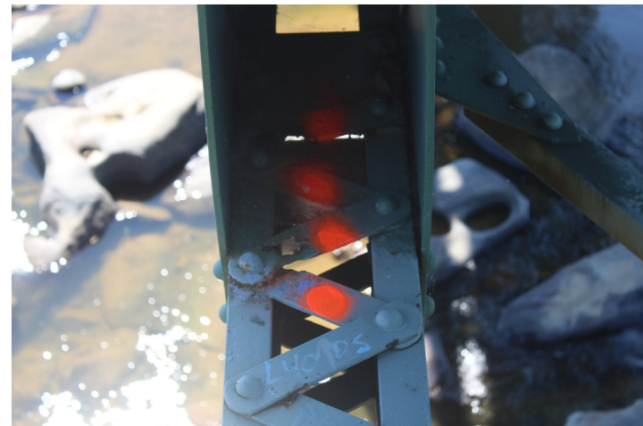
TYPICAL 100% SECTION LOSS OF LACING BARS
