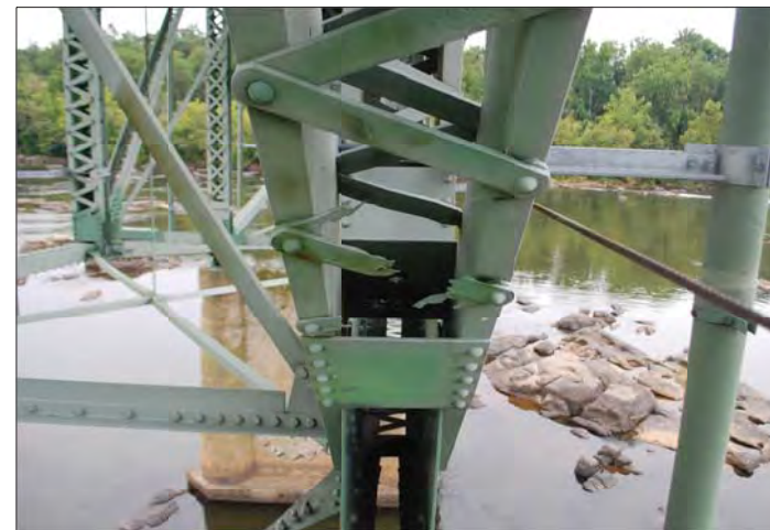
TYPICAL 100% SECTION LOSS OF LACING BARS AND BATTEN PLATES
