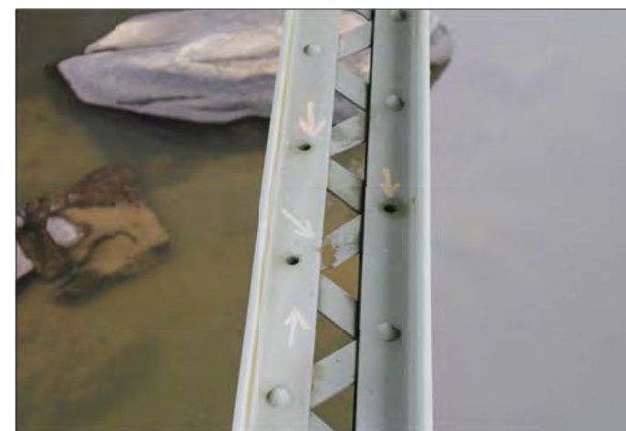
TYPICAL SECTION LOSS OF LACING BARS AND MISSING RIVETS ON TRUSS LOWER CHORD
